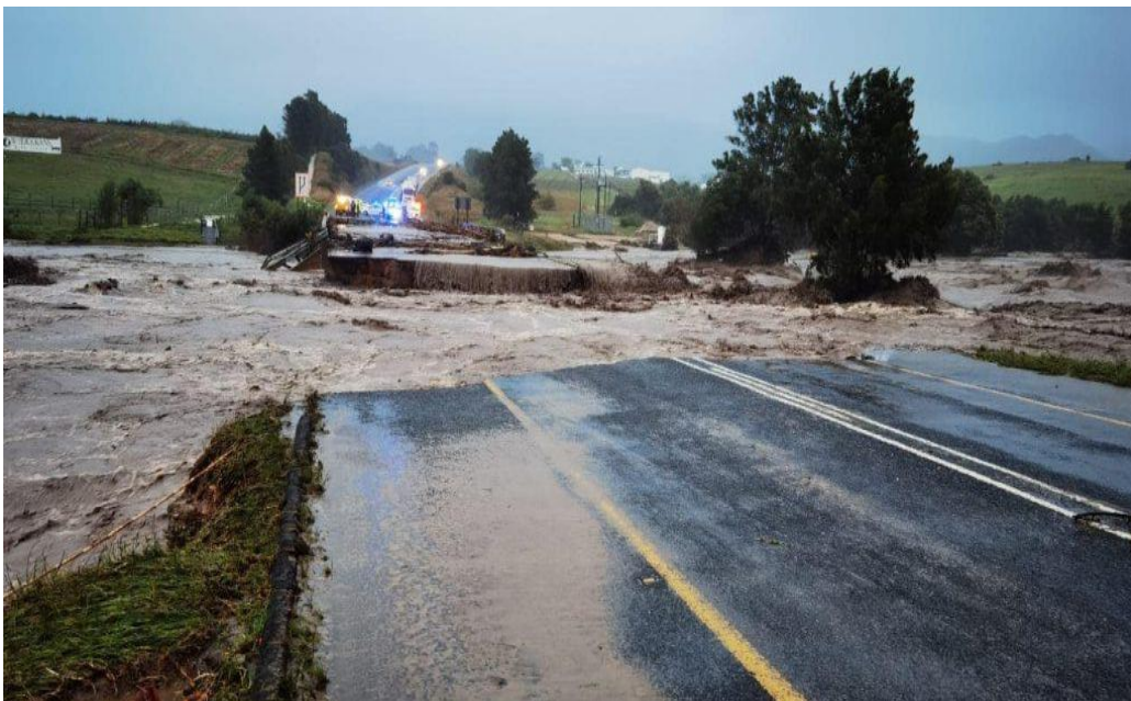
Bot River destruction of N2 Highway near small town of Bot Rivier (Source: Overstrand Municipality)
