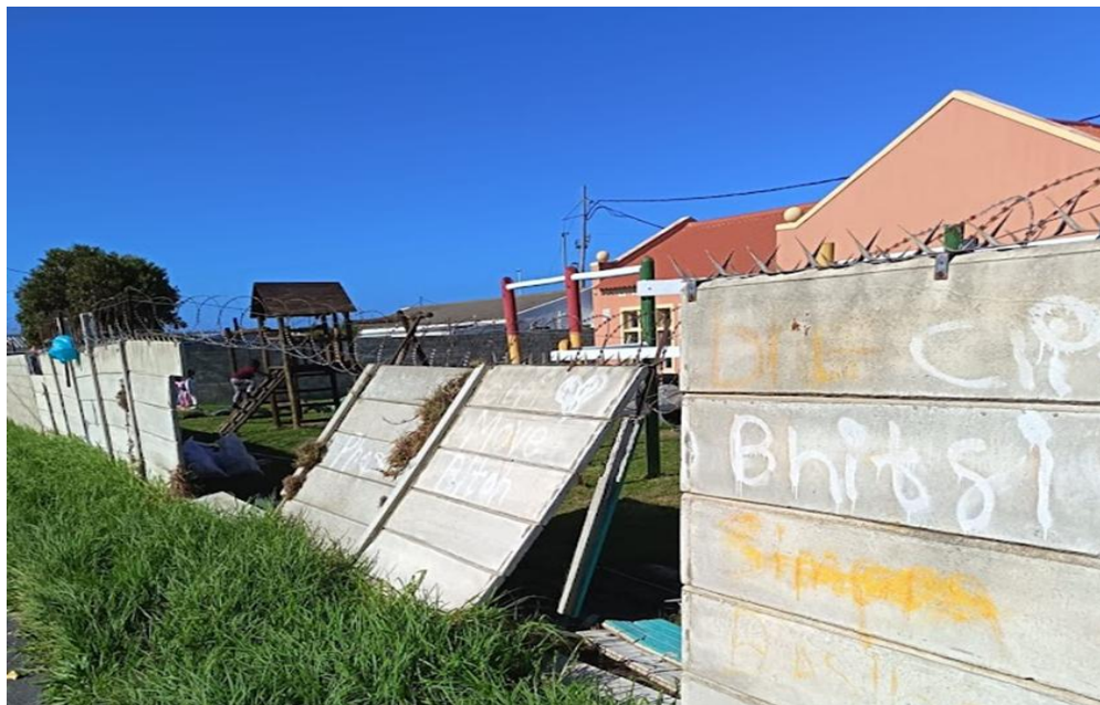
Nomzamo School perimeter wall after early-May 2026 storms
